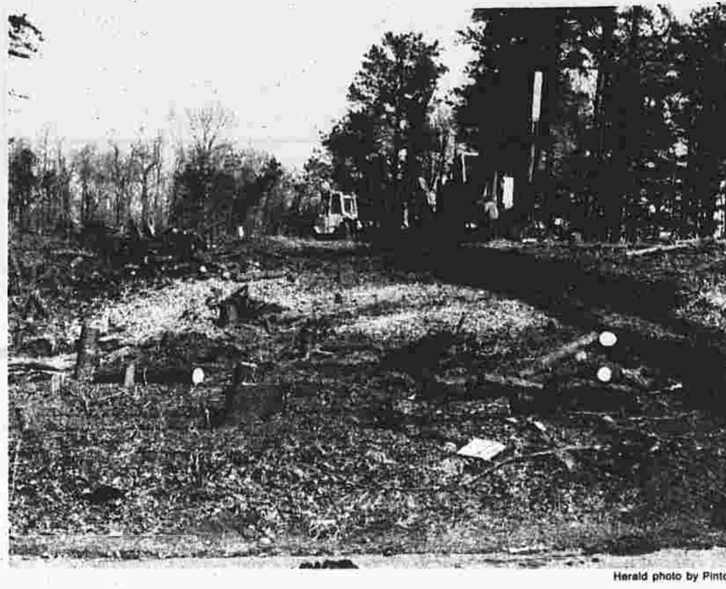
Work has begun on rough grading for the town's proposed water treatment plant. Frank Kapala and Son, excavators of Glastonbury, has the contract for the work.
